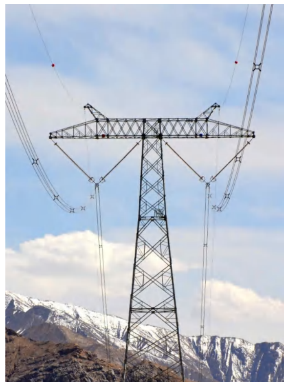
±400kV DC Qinghai-Tibet Project
