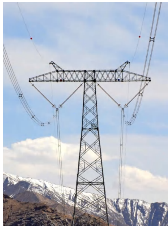
± 400kV DC Qinghai-Tibet Project
