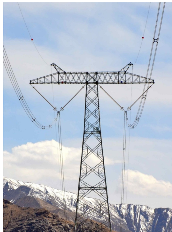
±400kV DC Qinghai-Tibet Project
